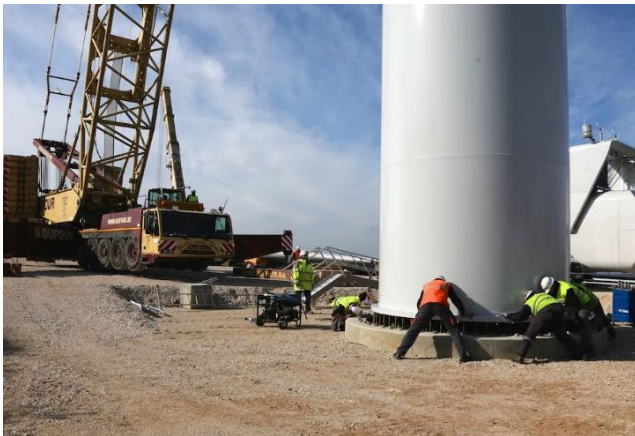
Source photo : Q ENERGY France
