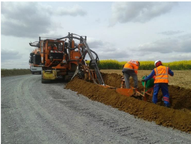
Source photo : Q ENERGY France
