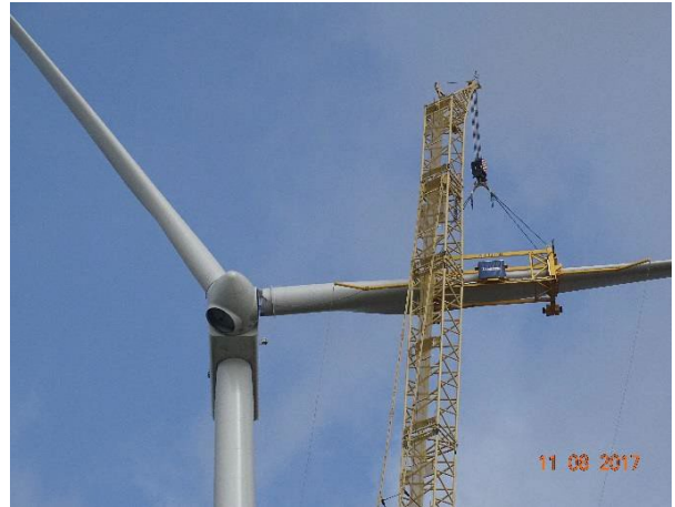
Source photo : Q ENERGY France
