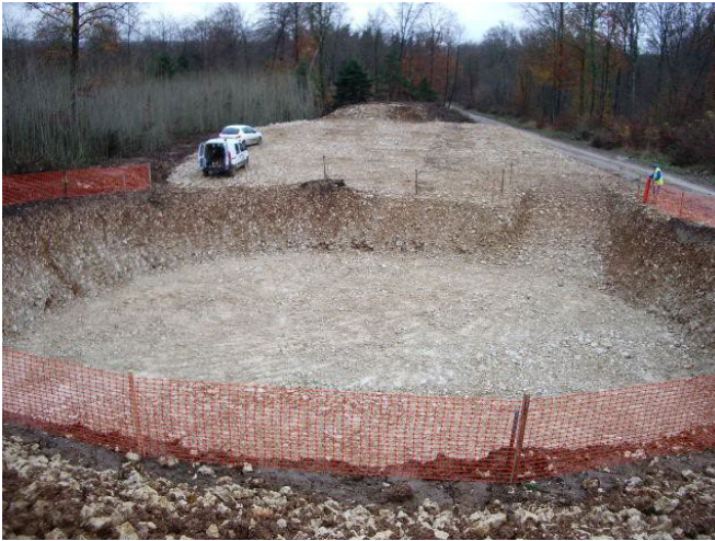
Source photo : Q ENERGY France
