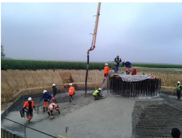
Source photo : Q ENERGY France
