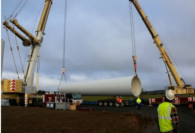
Source photo : Q ENERGY France
