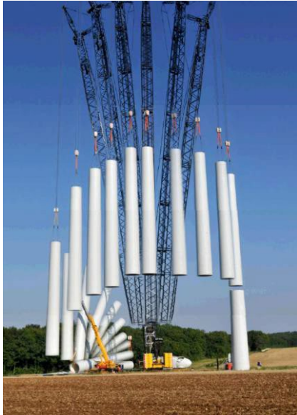
Source photo : Q ENERGY France
