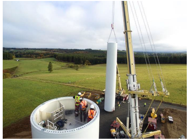
Source photo : Q ENERGY France
