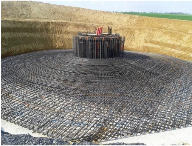
Source photo : Q ENERGY France
