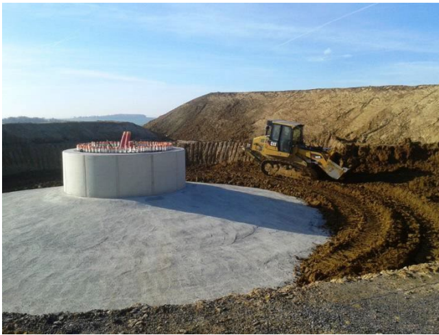
Source photo : Q ENERGY France
