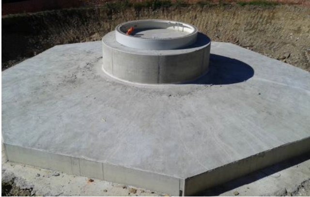
Source photo : Q ENERGY France
