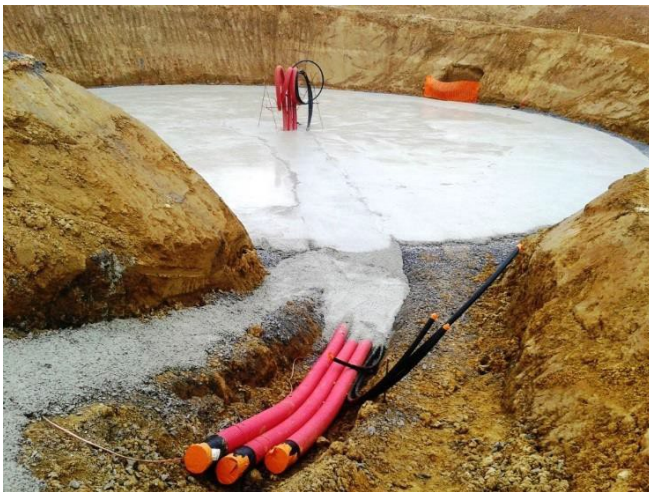
Source photo : Q ENERGY France
