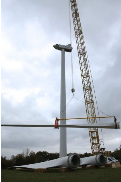
Source photo : Q ENERGY France
