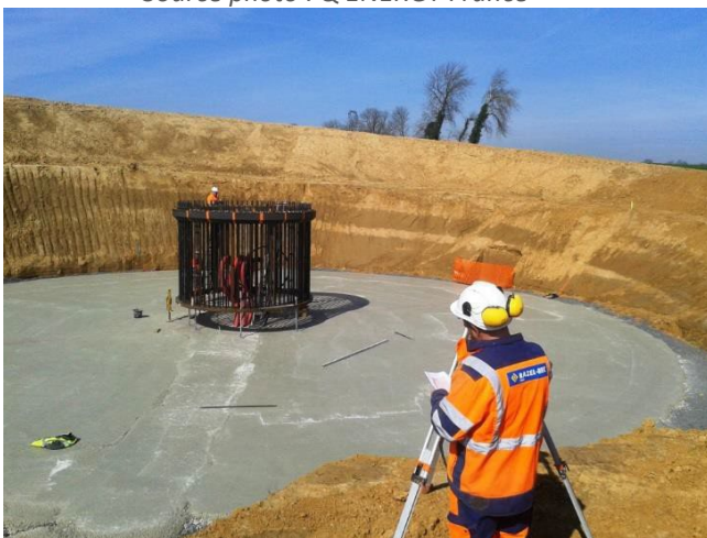
Source photo : Q ENERGY France
