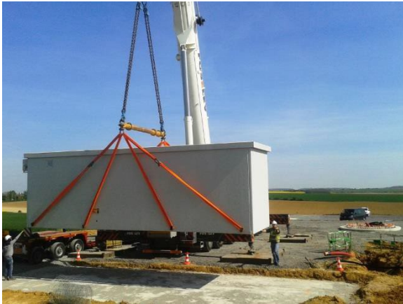
Source photo : Q ENERGY France
